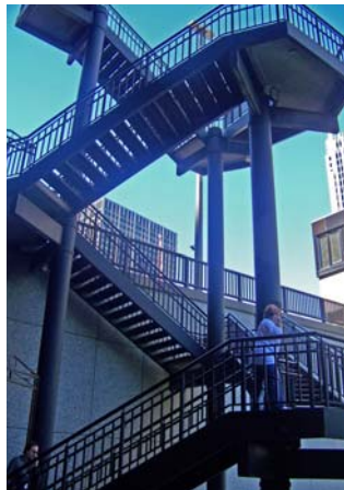
Currently, the Riverwalk is not accessible by people with disabilities. Working with the Mayor's office for people with disabilities, a series of access improvements were developed for this plan.
