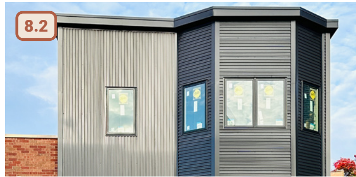
✗ Figure 50. Unacceptable reconfiguration of upper floor window openings
