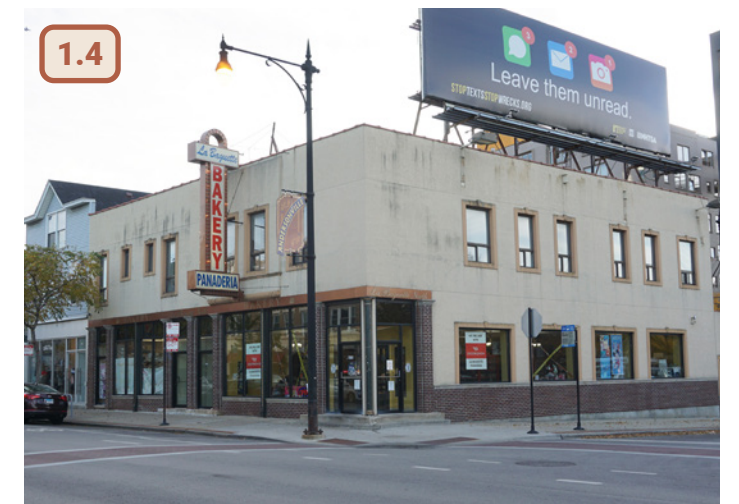
Figure 33. Unacceptable cladding over existing masonry
