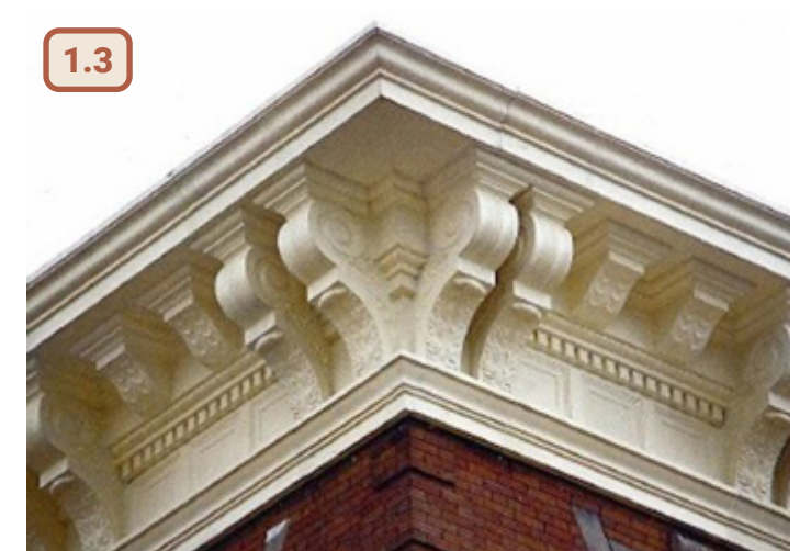
Figure 32. Acceptable substitute material: glass fiber reinforced concrete (GFRC) for terra cotta
