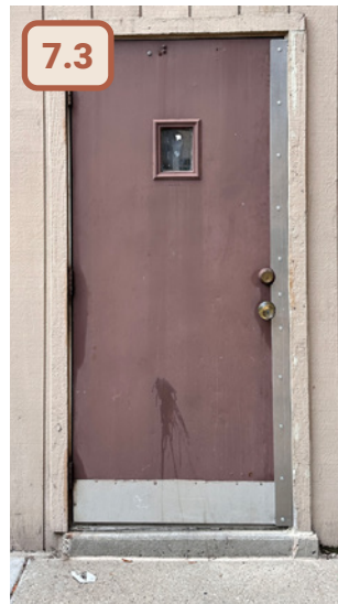
✗ Figure 46. Unacceptable example of a flush door
