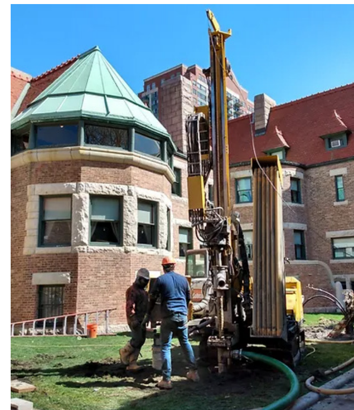
Figure 181. Example of geothermal energy being incorporated into a historic building (National Endowment for the Humanities)
