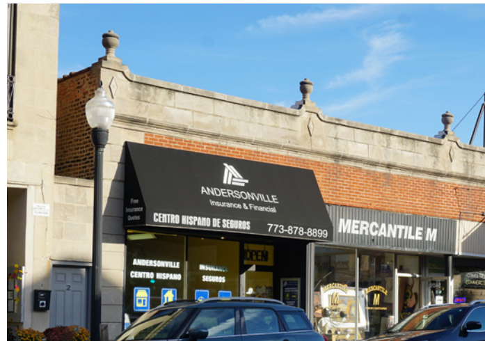
✗ Figure 186. Unacceptable example of replacement awning as it is not located within the existing masonry opening
