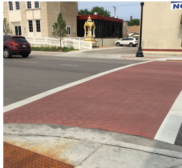
Figure 52. Enhanced crosswalk materials - Thermoplastic (Source: IDOT)
