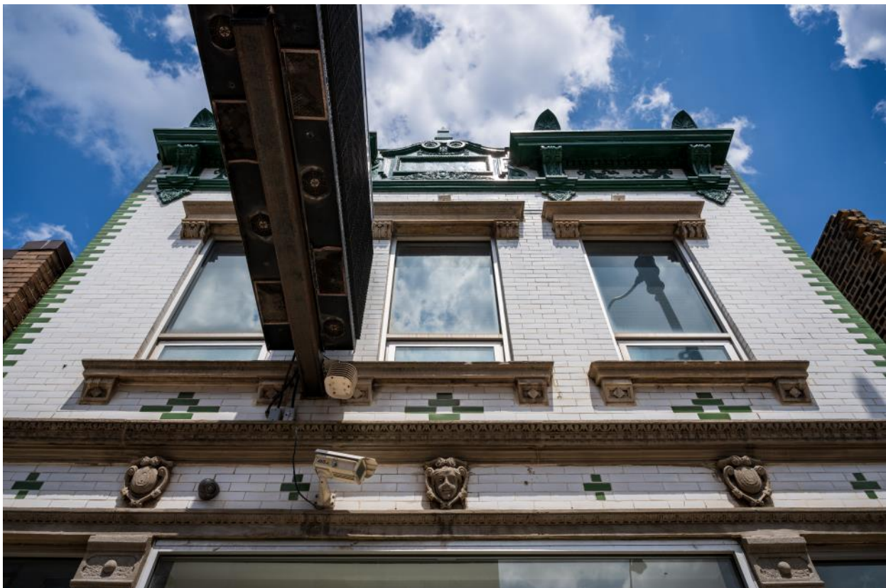
Below: Bedford limestone trim includes shields and mascarón between belt courses above the first floor and window hoods and sills at the second floor. The pressed-metal cornice projects significantly from the top of the façade. (Photo by Patrick Pyszka)
