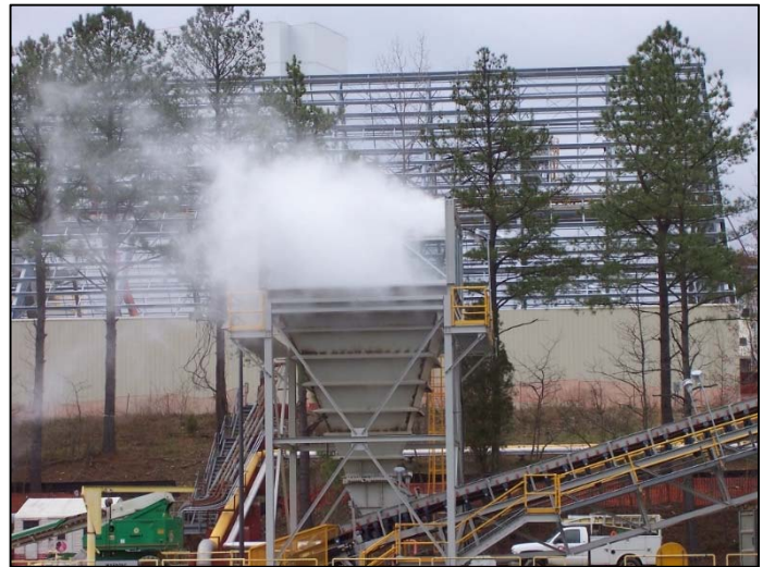
Figure 8: Photo of a dry fog system with wind fencing on a receiving hopper at a coal power plant.
