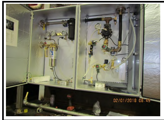
Photo # 4 Pressure gauges and flow control for DCI Dry Fog Truck
