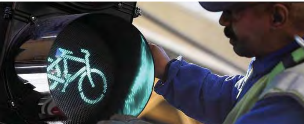
A city worker installs a bicycle signal head on Dearborn Street Courtesy Chicago Tribune, 14 December 2012
