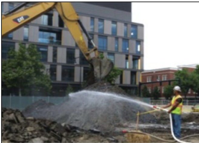
Photo: Vapor Suppression
